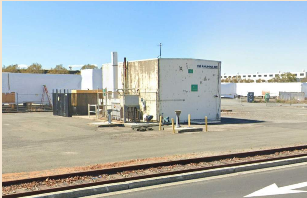
Existing DOM 4 Pump Station
