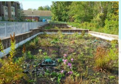
Stormwater retention using bio-retention Basins
